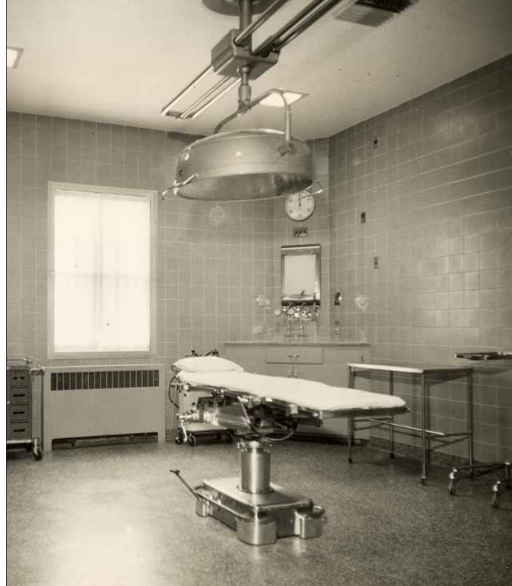
The addition of air conditioning was central to the modernization of operating suites in the 1950's.
